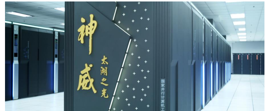
Supercomputer, data center (2020s)
